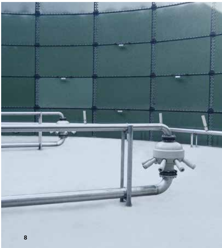
Ejectors and mixing nozzles for aeration and complete intermixing in an SBR reactor
