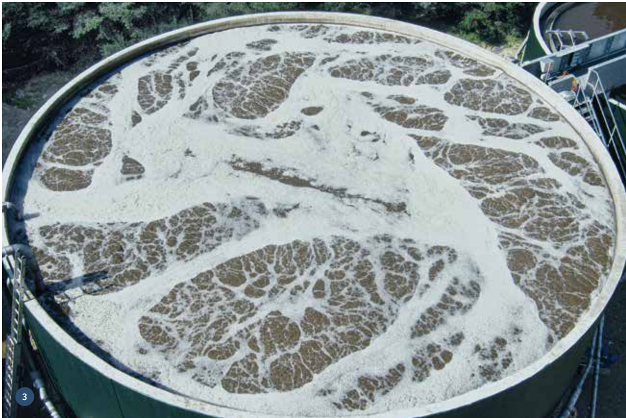
3/4) 1 200 m 3 aeration tank from a paper mill in Germany
