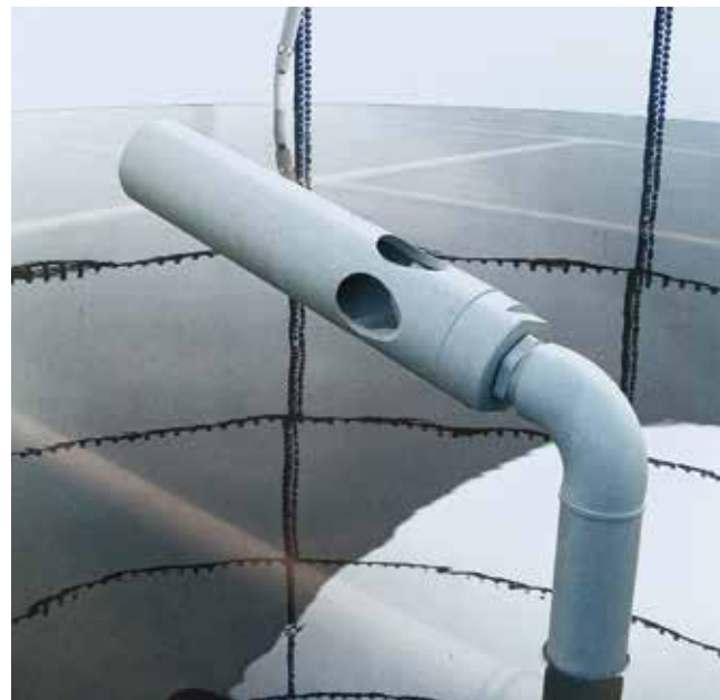
Mixing nozzle in a denitrification
