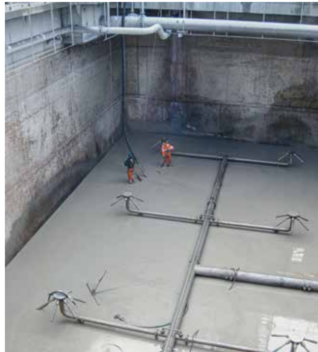
Oxygen transfer system in the aeration tank of the Gebr. Lang GmbH paper mill in Ettringen, Germany. The six-path ejectors are supplied with gaseous oxygen from a stationary tank system.
