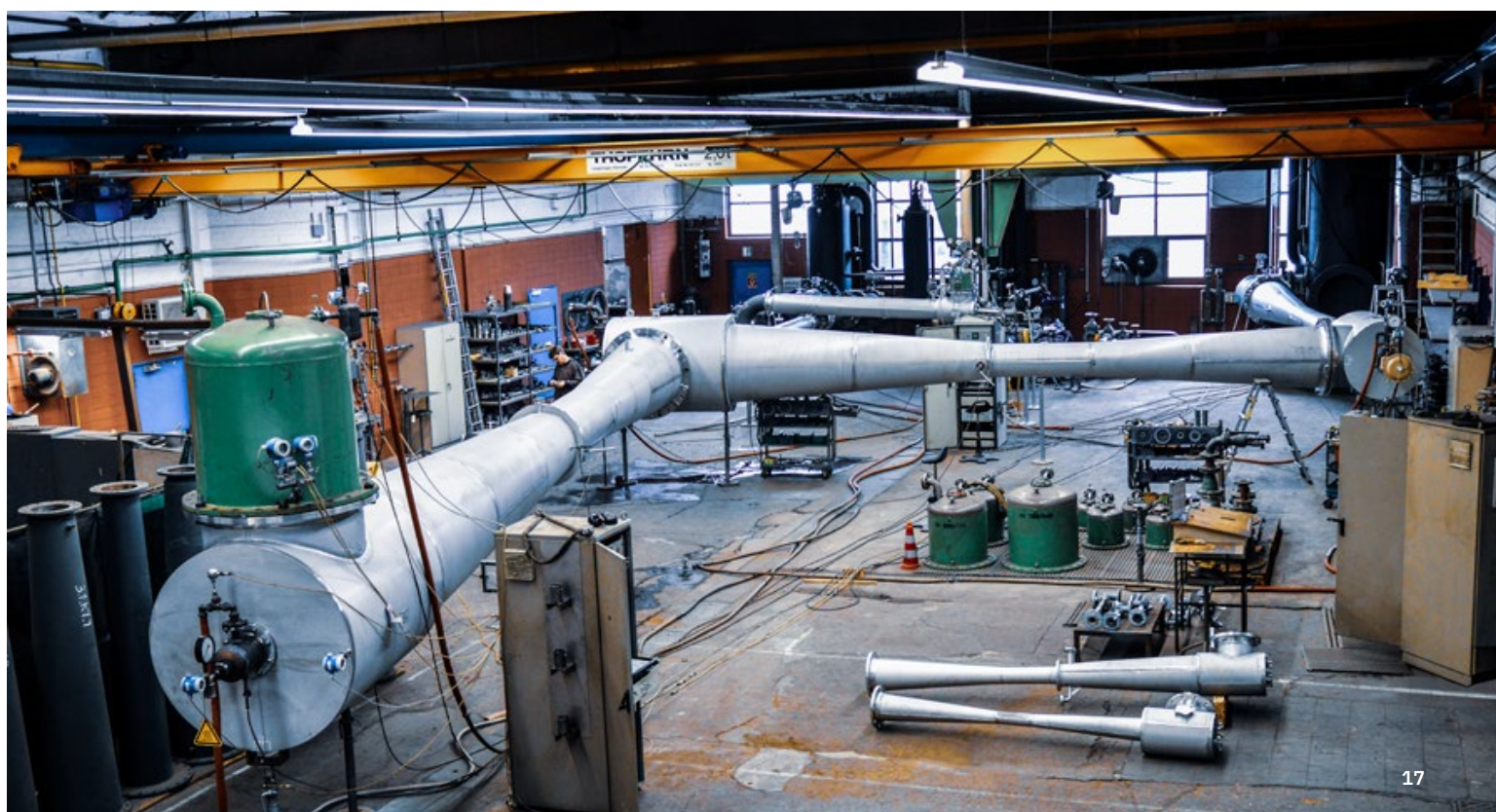
Three-stage steam jet vacuum ejector on the Körting performance rig
